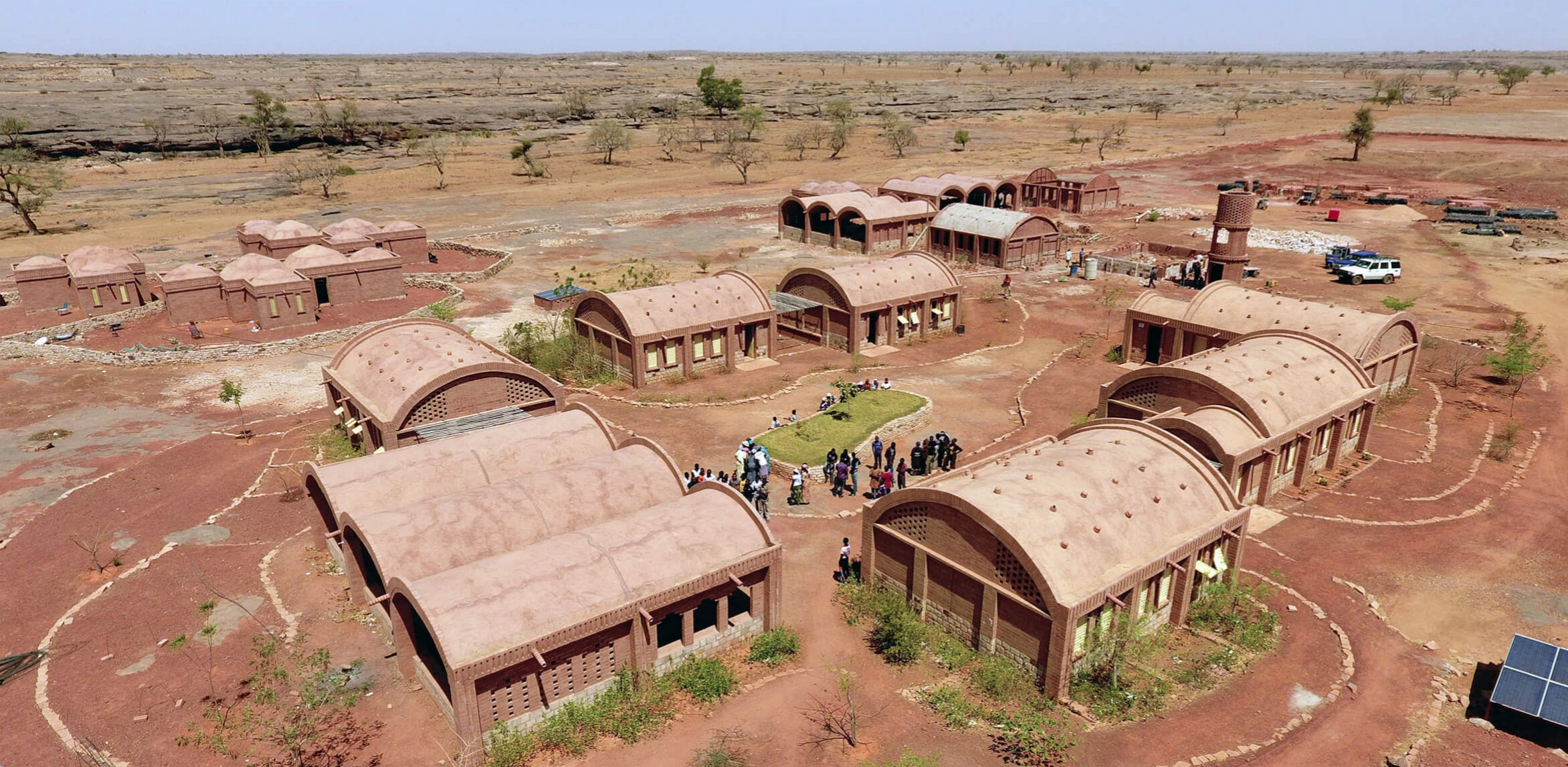
Practical Training College Sangha, construction of the second cluster, 2018, Photo by LEVS architecten
